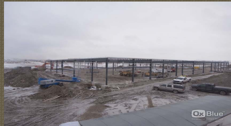
Watford City: 118,000-square foot commercial shopping center
